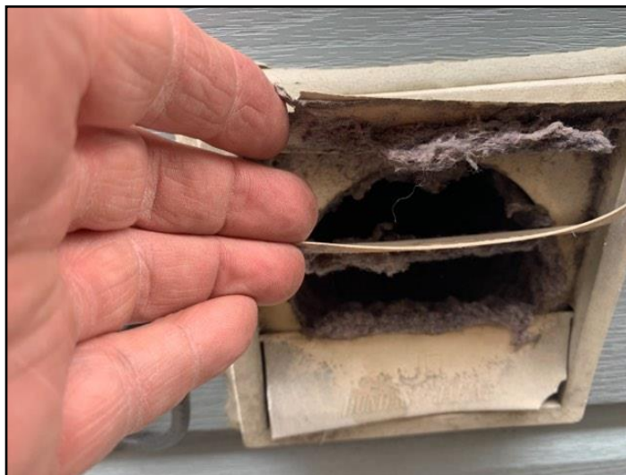
24. Dryer vent obstructed
