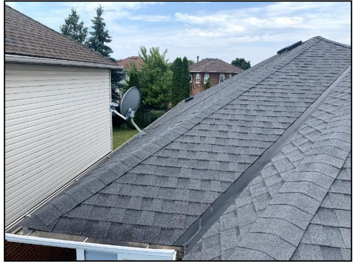
7. Doesn't widen at bottom
