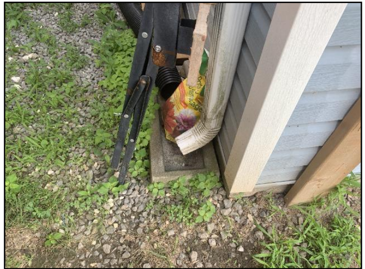
10. Should discharge 6 feet from building
