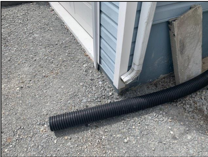
9. Should discharge 6 feet from building
