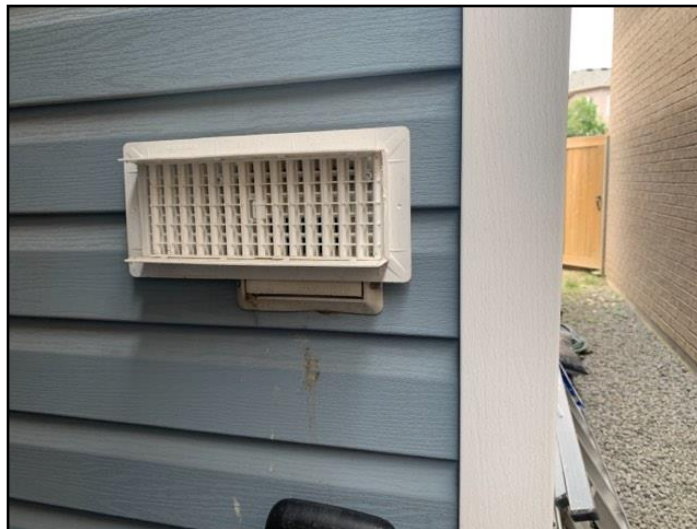
23. Inadequate air movement
