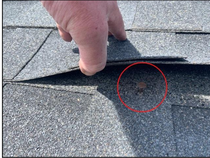
5. Missing, loose or torn
